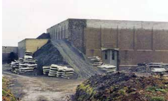
Bomb-proof slabs and several feet of shingle being removed from the roof in 1990. Photo Sandy Windwick
